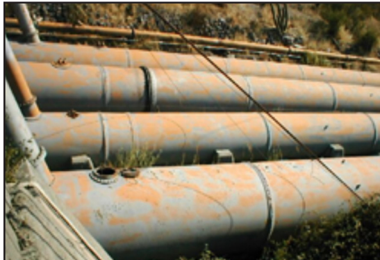
Penstocks viewed from outside
